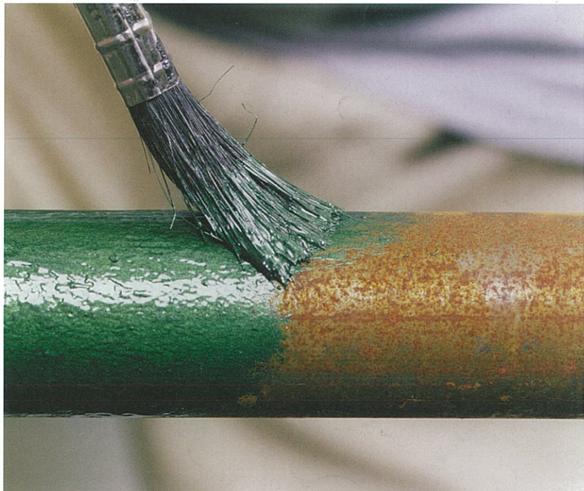
Fig. 9.5. Special metal paints can provide an easy-to-apply, durable finish. Some can be put straight on to metal, even rusty metal once the worst rust has been removed. (Steve Williams)
