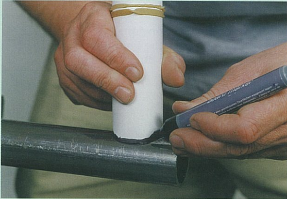
Hold the end of the card tube against the steel tube to be joined to, and mark on the card the approximate shape of the steel tube. (Steve Williams)
